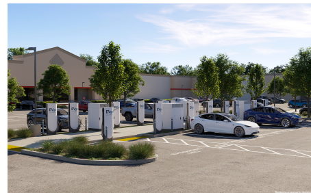
EVgo plans to install “EVgo Superchargers” across the country to make fast charging even more accessible and widen NACS charging options
