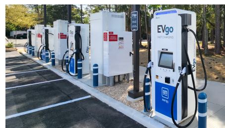
A prefabricated EVgo station at Regency Group's Mandarin Landing in Jacksonville, Florida.
